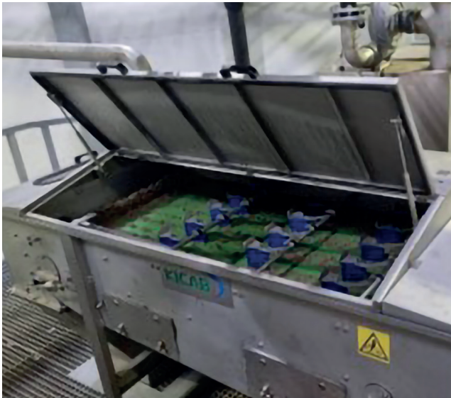
Sludge processing unit at Kjærrelva.
