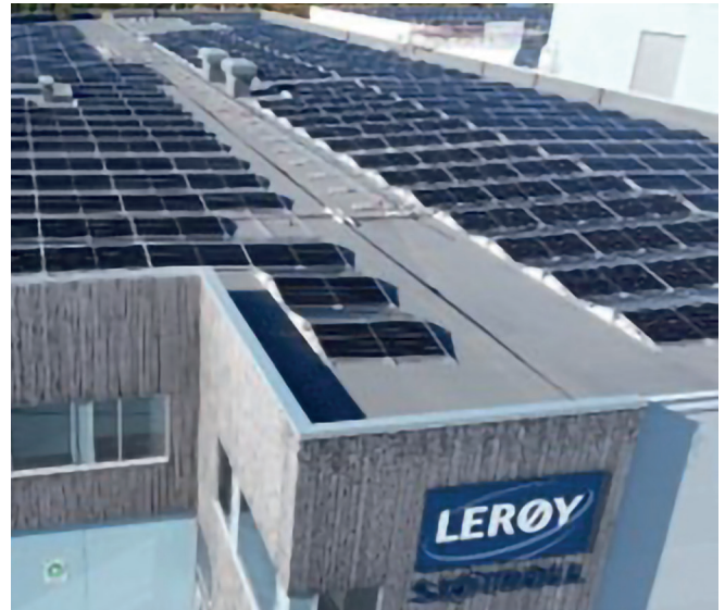
Solar panels at Kjærrelva.
